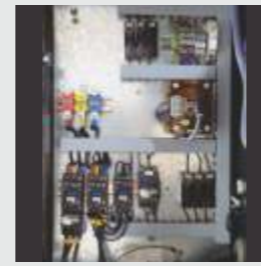
Electrical Cubicle Monitors Power Management
